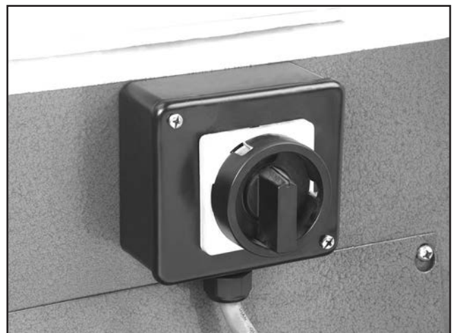
Figure 10. Master power switch.
