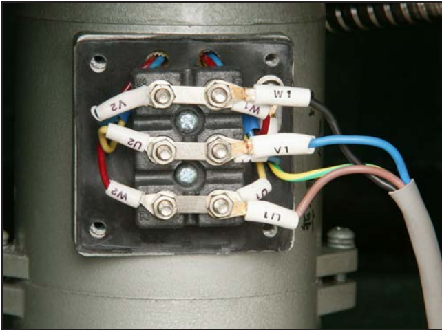
Figure 112. Pump wiring (M2).
